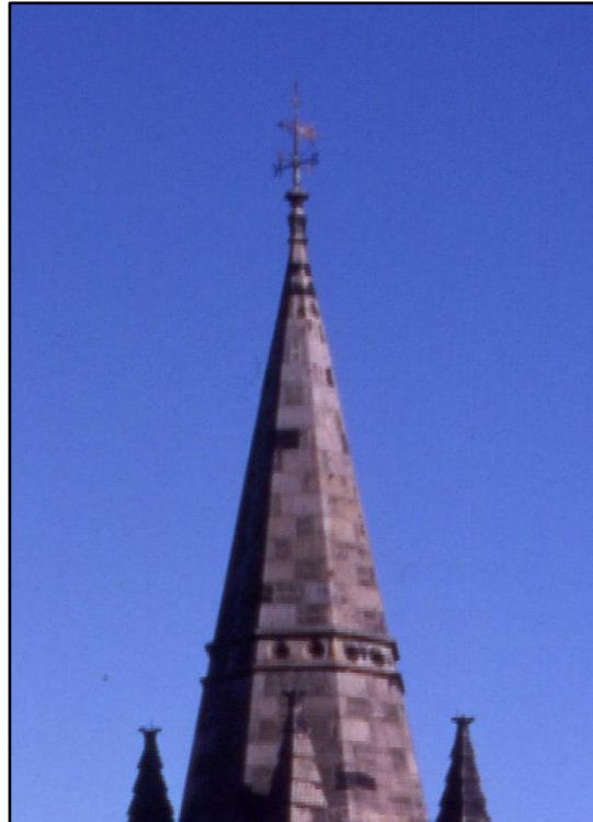
This 1995 photo shows the weathervane rising precariously above the top of the steeple.
